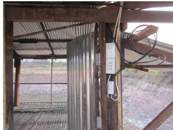
The electricity system at the coop
